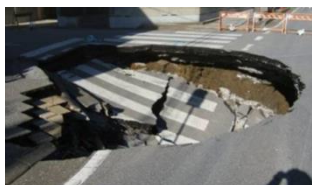
Fig.1 Sinking by cracks
